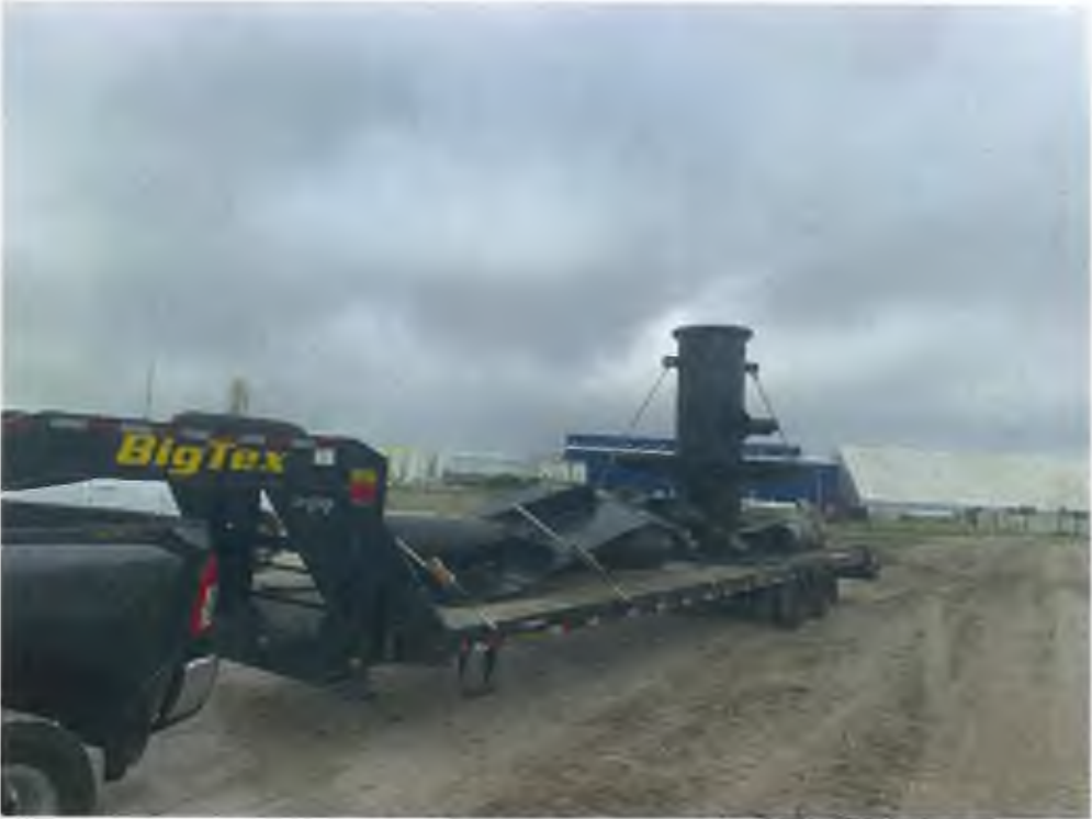
Photo 12 - Received 18" spool (flanged tees), 18" liner penetration, 6" liner penetration, and 36" HDPE manhole structure
