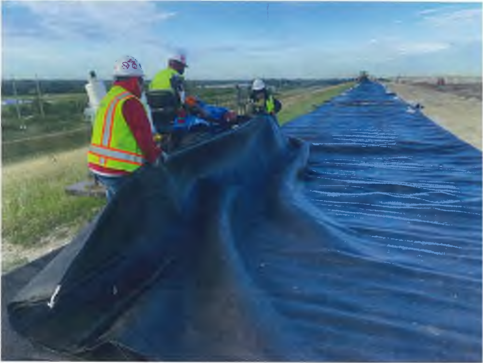
Photo 11 - Sewing Three Additional Panels of High Strength Fabric for Seam Repair Plan
