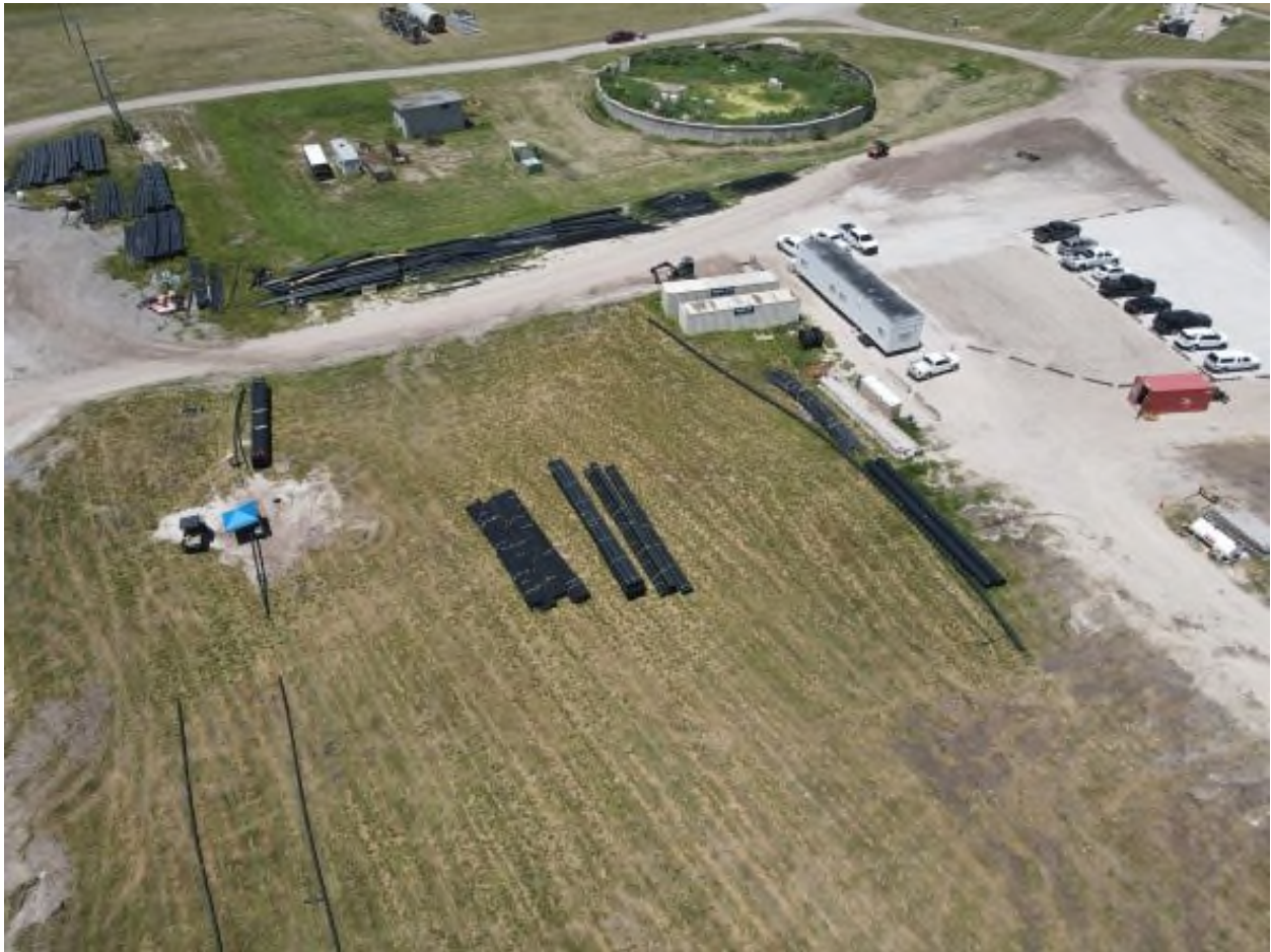
Forgen's modular office, employee parking lot, and laydown yard for supply and pipe storage.
