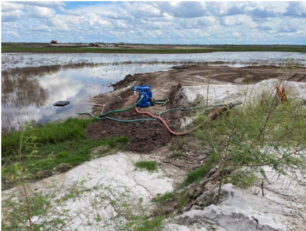
Photo 7 – Dewatering Pump - Sump Area
