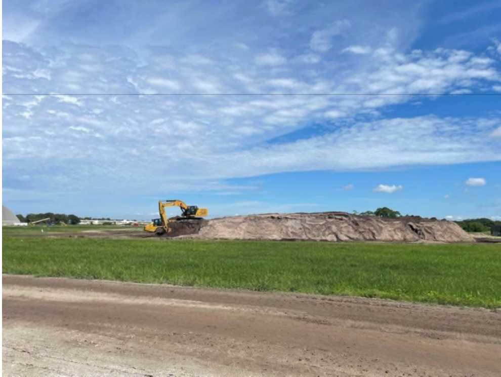
Photo 10 – Hauling Soil from the Stockpile to Place 1-foot Thick Layer of Soil
