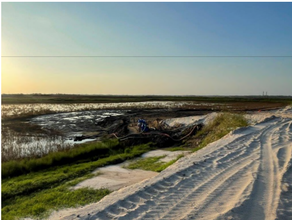
Photo 8 – Dewatering Pump - Sump Area
