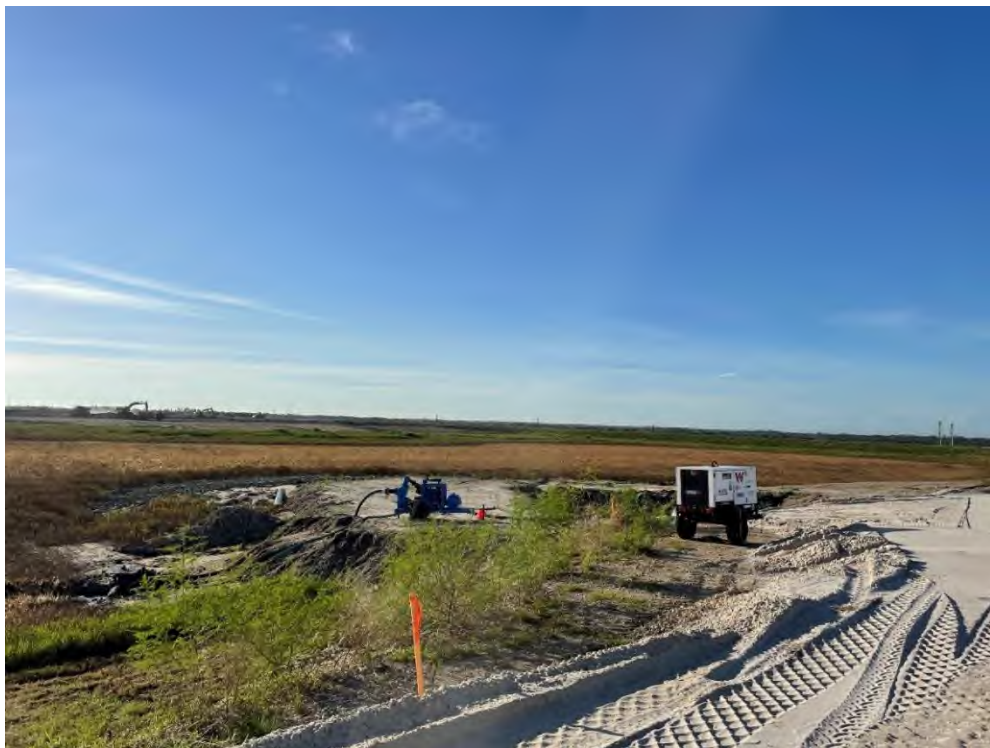
Photo 8 – Dewatering Pumps in Sump Area
