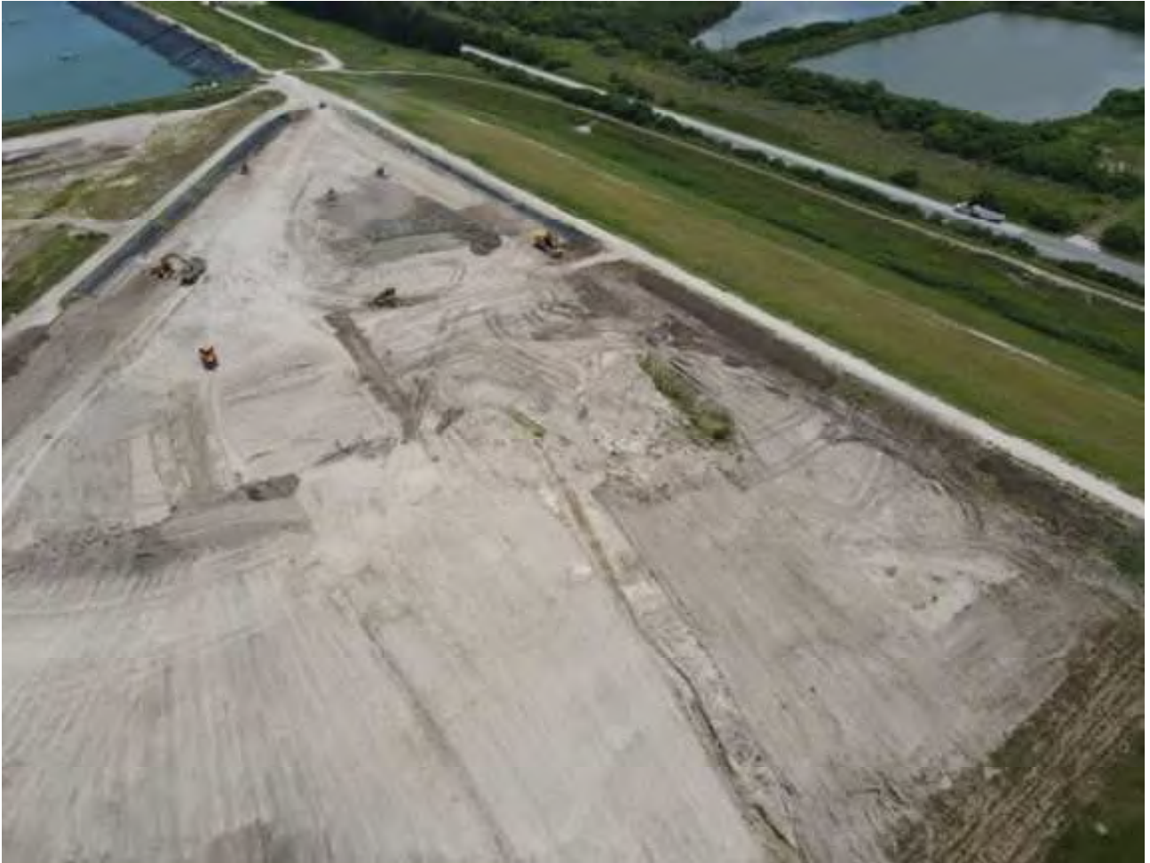
Crews and machinery contouring the inside of OGS-S to conform to the Stormwater Management Plan.
